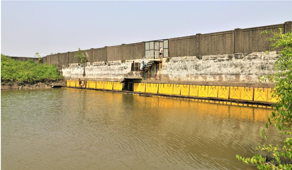
Image 1: Tide gate on the creek at Panje Wetland. Image shows upper 35 flip valves while lower 35 valves are submerged. Currently these flaps are open allowing tidal water to flood the wetland. The closer of these flaps will kill the entire wetland
